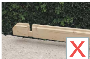
Concrete base running out of level by more than 10mm.
