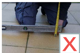
Slab base has a water run-off allowance making the base run out of level by more than 10mm.
