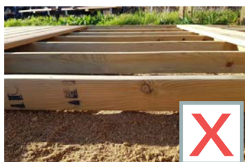
Base substrate not a solid material making the base unable to support heavy structures.
